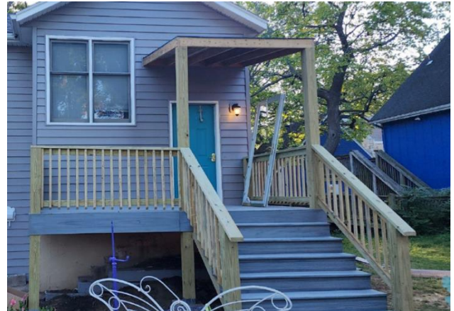
Exhibit 5: Newly constructed front porch encroaching 13 feet into required setback.
