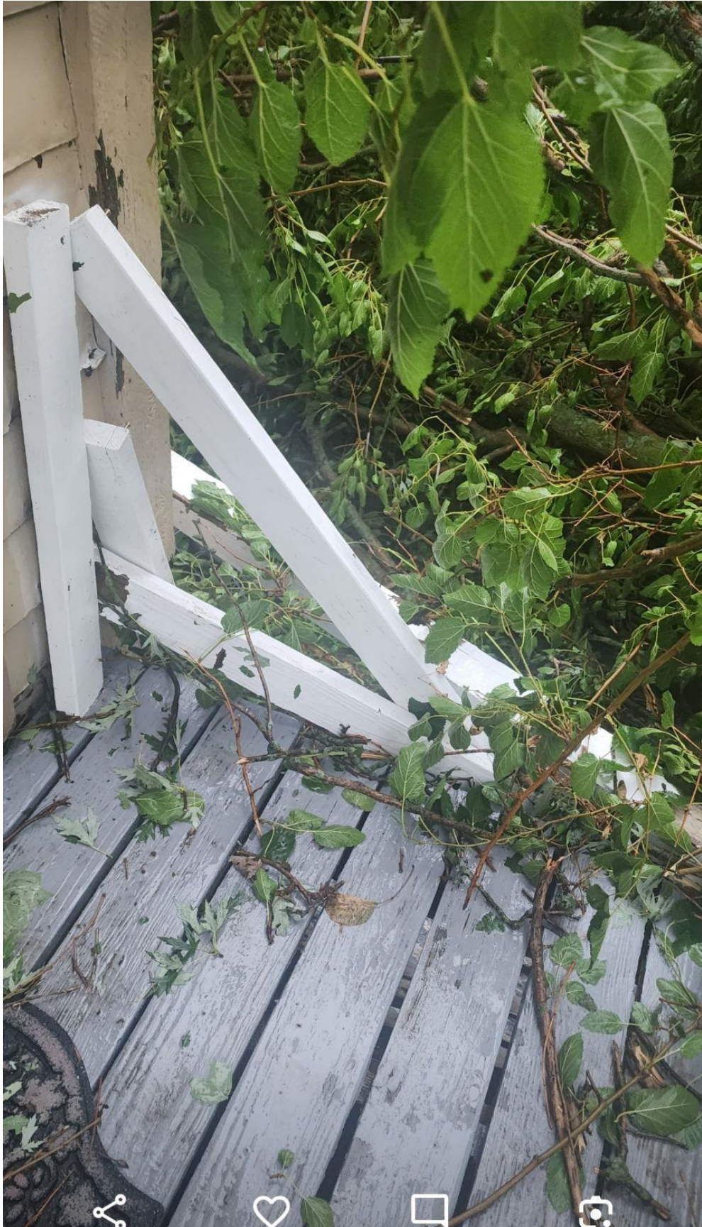
Picture of storm damage provided by applicant
