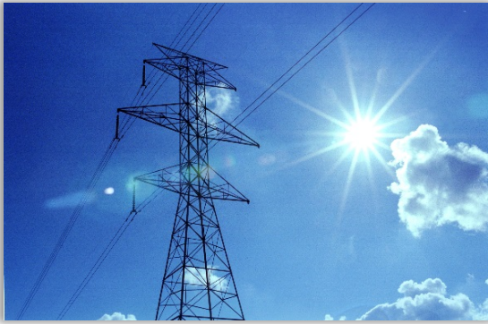
High Voltage Transmission Lines
